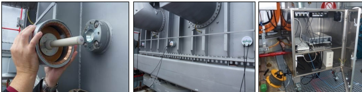
Fig. 1. Left - sensing head, middle - sensing heads mounted on the transformer, right – assembly of the diagnostic system in shielded box.
